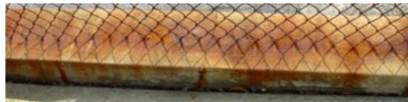
Concrete Curb with Severe Rust Stains Before SB 2301
